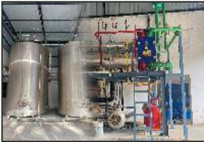
Strengthening milk procurement eco system by installing latest technologies with ammonia plant at our Kutiyana Chilling Centre and Bhavnagar BMC
